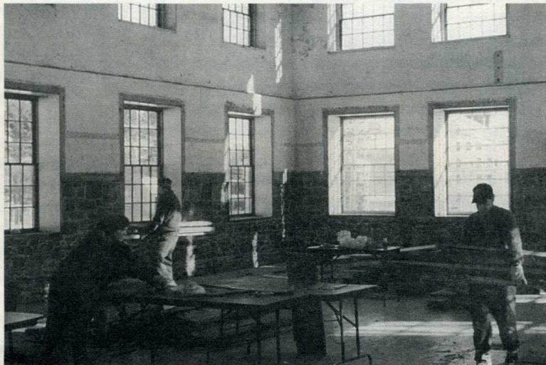
Volunteers at work in the Stone Mill Building in preparation for Precious Gospel Kindred exhibit opening June 28th. Non-Shaker wainscoting was removed and windows restored to provide a more authentic and comfortable exhibit gallery.
