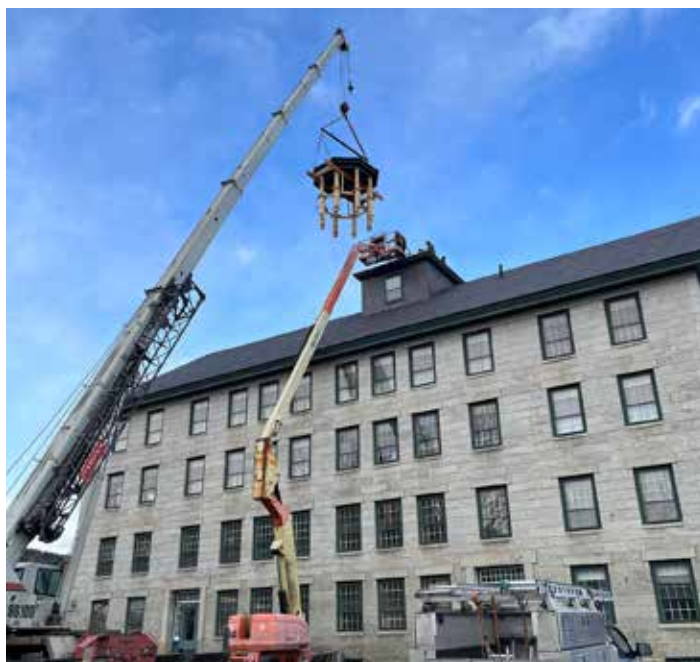
The belfry and bell return to the roof of the Great Stone Dwelling.
