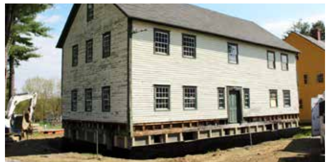
Early April 2024 Brethren's West Shop is lifted 5 ft off its foundation. Original Shaker chimney bases are restored and receive new granite caps. Late May 2024 the building is back on its new foundation. Photos: Susan Brown 2024
